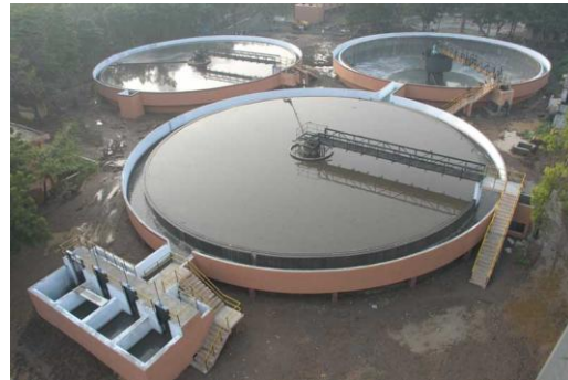
Pr. Settling Tank
