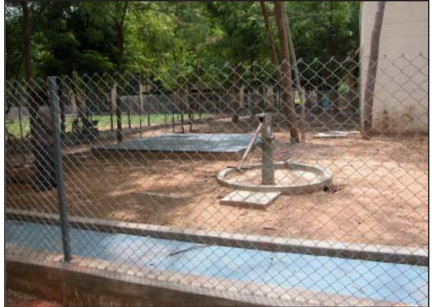
Gravity filter connected to the tube well - Recharge system in Workshop area - ▲
