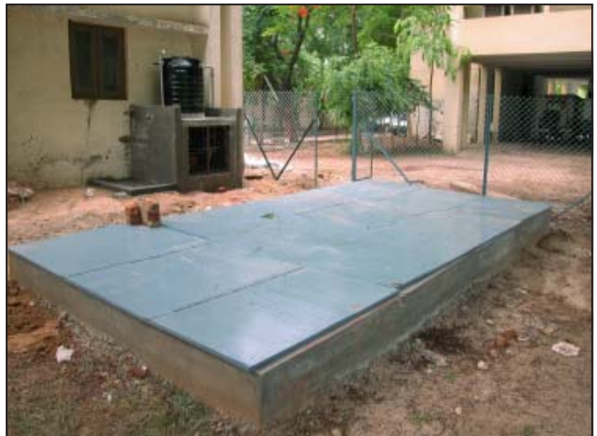
Gravity filter covered by MS Steel sheet fixed to steel Grill - Minimum maintenance ▲
