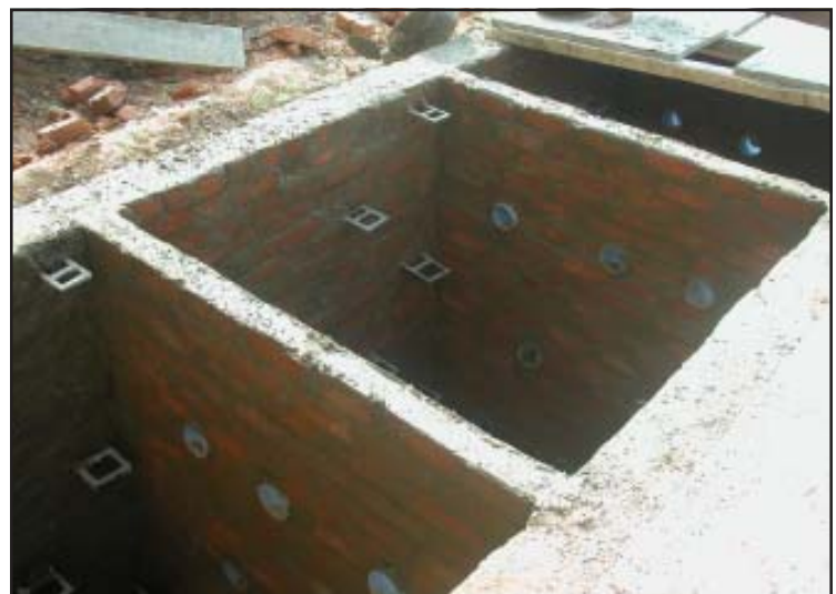
Openings in Horizontal Filter - GJI
