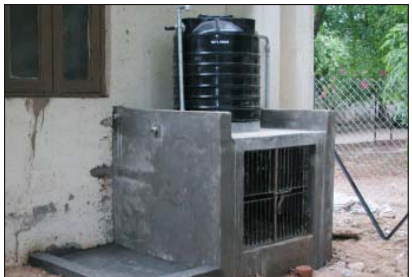
Reuse system -Provision of Dispenser tank ▲
